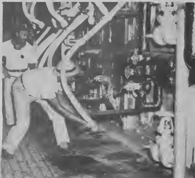
THE NEW boiler is set to go! Fireman Cyril Cayol holds the torch ready as Waterfeller Alfred Bishop adjusts the first of six burners. E BOILER nobo ta cla pa cende! Fireman Cyril Cayol ta parrs cla u e torch mientras Waterfeller Alfred Bishop ta abusta a premier burner.
